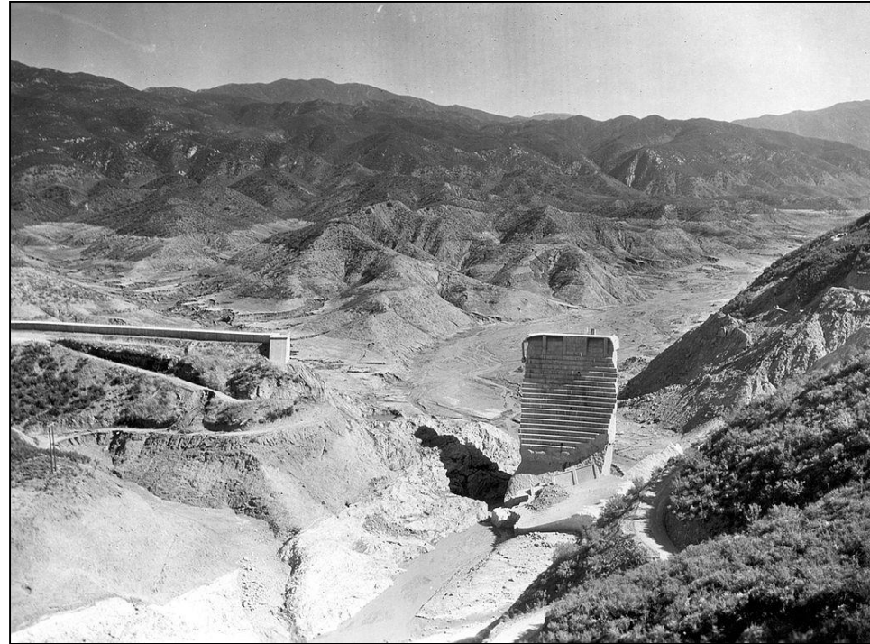
Dam failed due to defective foundation
