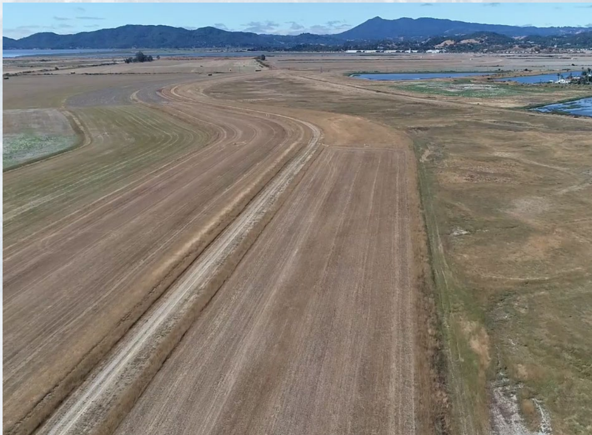
Drone footage of Bel Marin Keys Unit V new setback levee - Haley & Aldrich, July 2022
